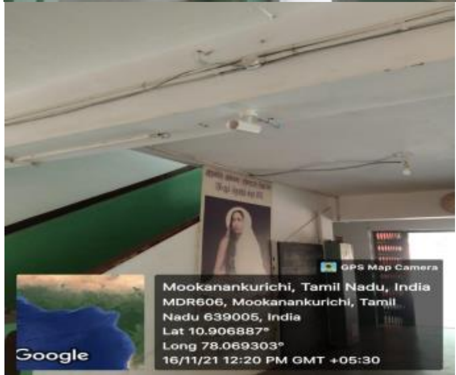
CCTV camera in prominent places
